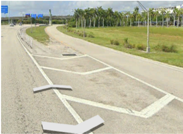
Figure 1: Informal Gore Gutter
